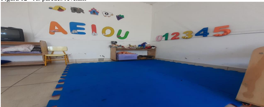
Figura 12 - As paredes revelam
